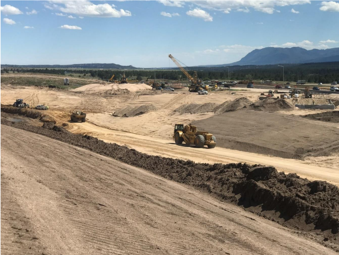
Dwire continues to move material, approximately 900,000 cubic yards. Topsoil is placed on the slope as it is finished (the darker material).
