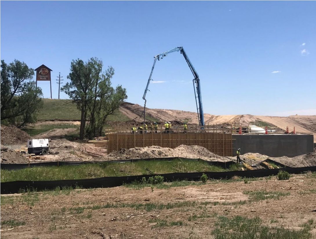
Box Culvert DO was poured on June 12 th . The new off ramp from Powers & from I-25 will cross the box culvert delivering traffic to North Gate Boulevard.
