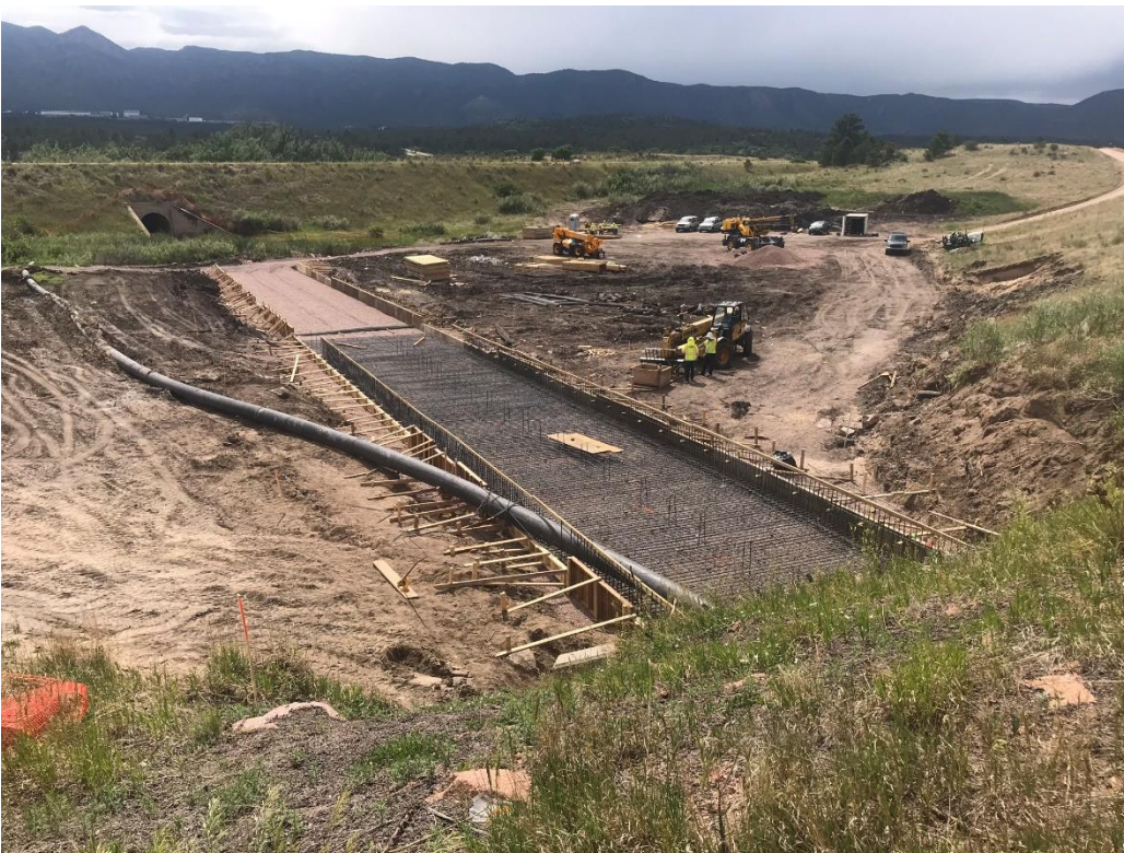
Work has started on box culvert AL, which is west of the Interstate. Rock is first installed to stabilize the subgrade. The bottom of the box is being formed.
