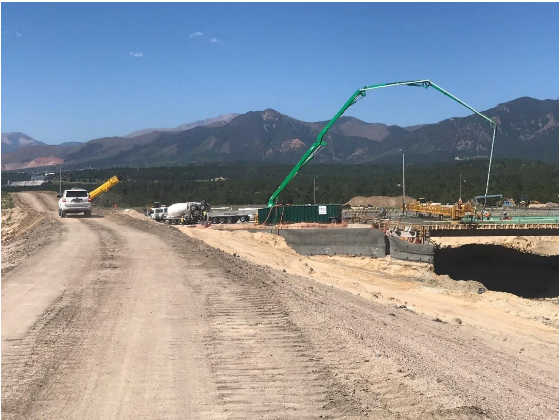
June 12 th , the deck is poured using a concrete pumper. Concrete trucks deposit concrete in the back of the pumper.
