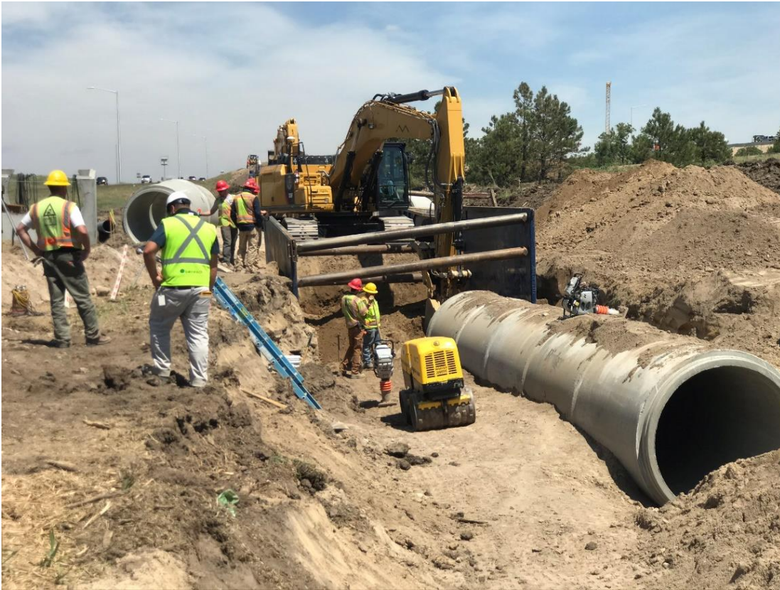
Redline construction has brought in a second crew to install the “B” line, which runs down the median of I-25.
