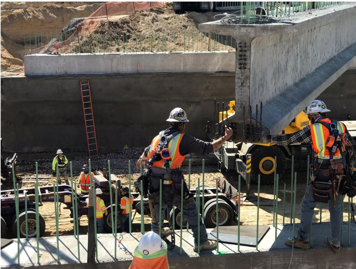
The girders are placed on an elastomeric bearing pads, which will evenly distribute the weight.
