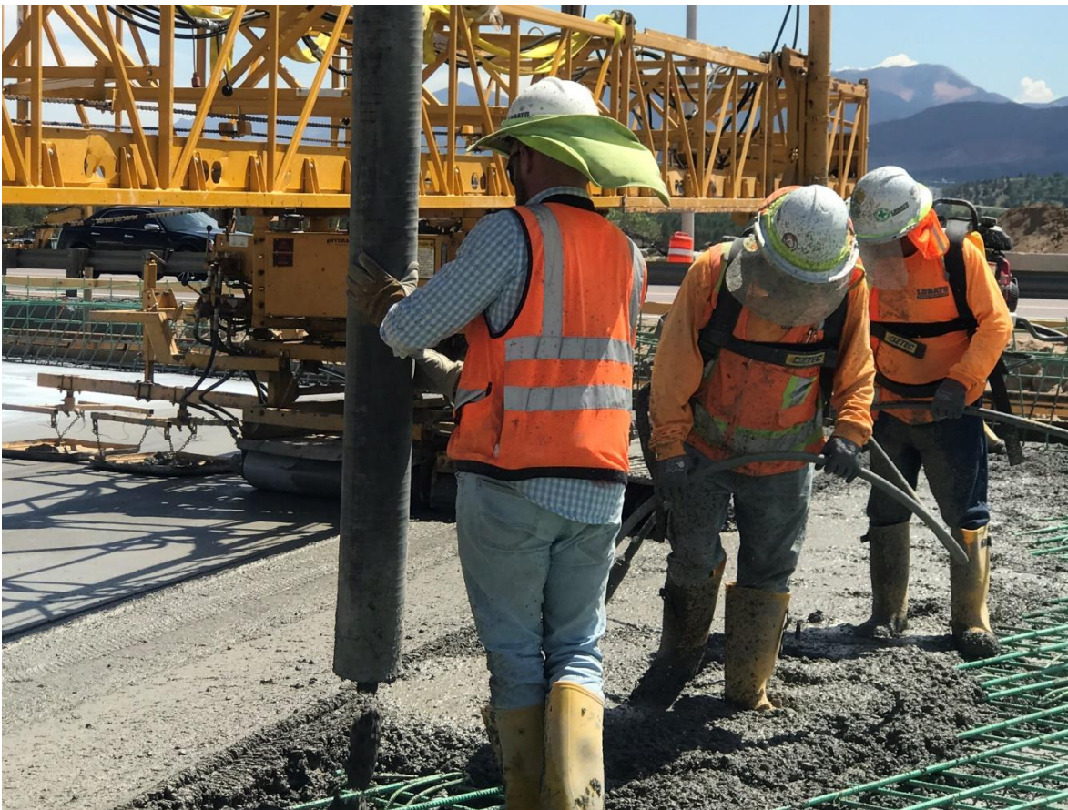
The concrete is pumped in front of the Bidwell Concrete Paver, then consolidated by vibrators.
