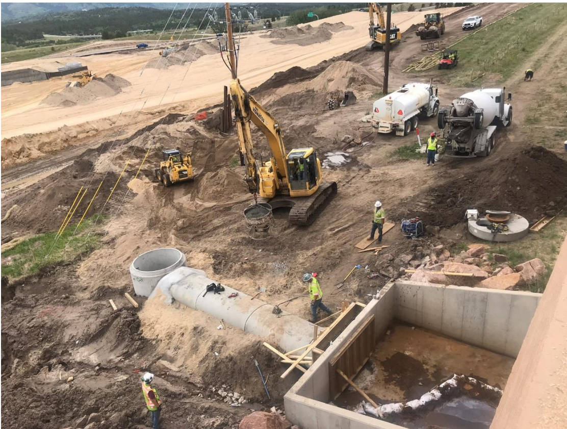
Wildcat is installing the “C” line, which will drain storm water from the Bass Pro Pond to Smith Creek.
