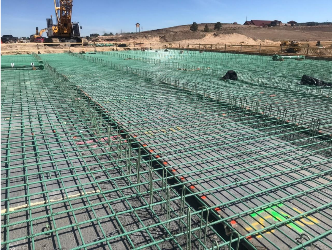
The reinforcing steel is placed. The steel is epoxy coated for corrosion protection.
