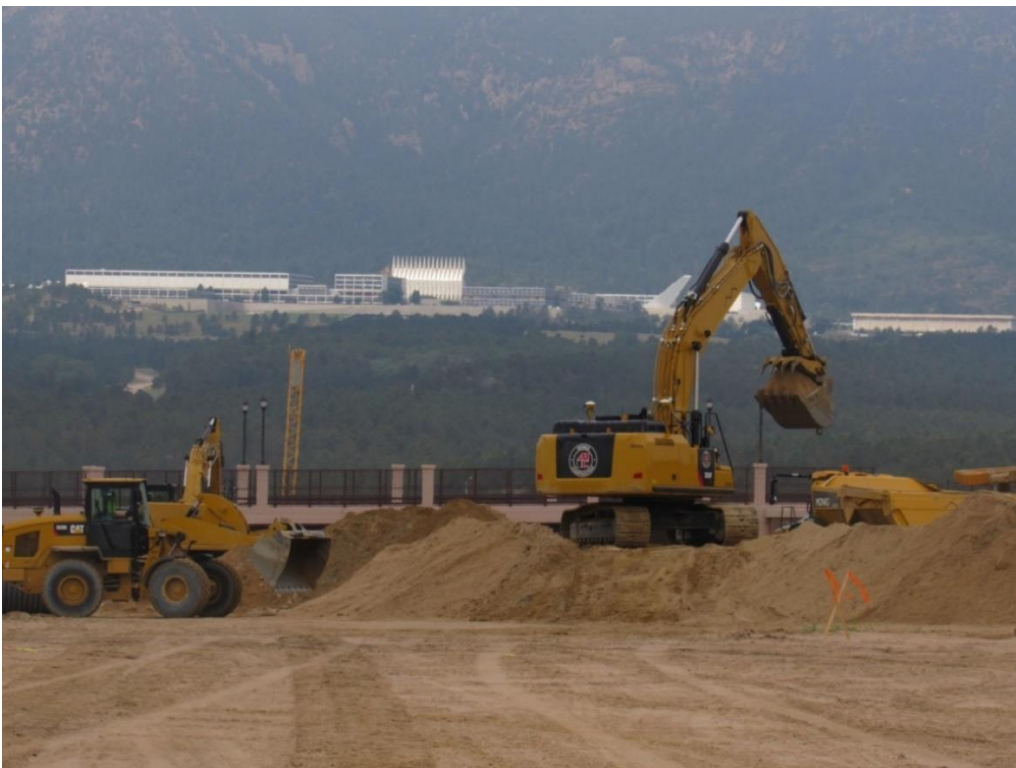
Redline Pipeline out of Monument, Colorado is installing storm sewer down the mainline of Powers. Redline is being assisted by R. E. Monks Construction out of Colorado Springs.
