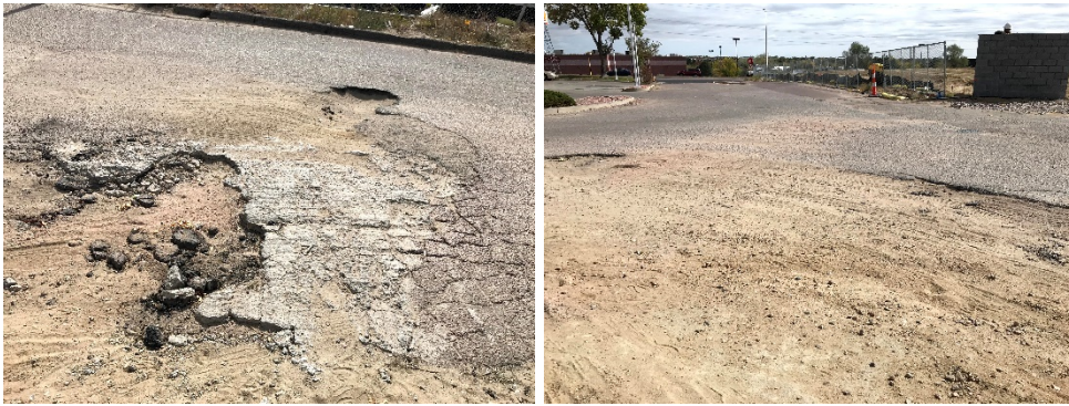
Figure 2. Poor Provision of Street Improvements
