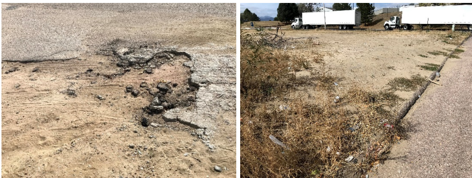
Figure 10. Deteriorated Pavement and Curbs and Missing Sidewalks
