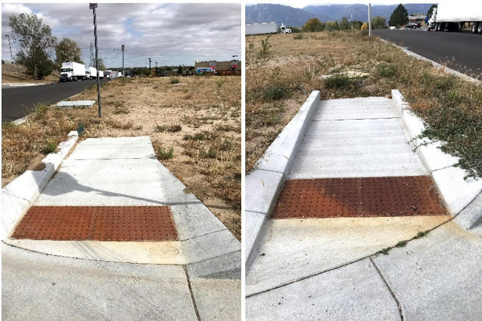
Figure 3. Lack of Sidewalks
