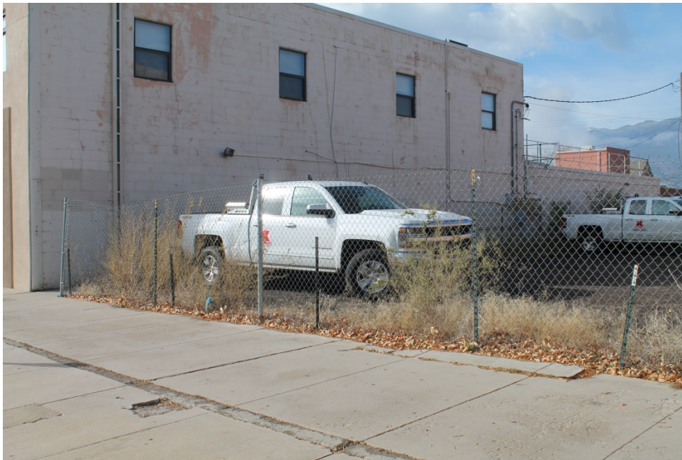
Figure 2-4 Deteriorated walls/fences; presence of trash and debris; trip/fall hazards; inadequate site maintenance; non-conformance to development regulations; deteriorated sidewalks in the right-of-way; dry debris a near structures; hazardous materials near structures (Photo 6)
