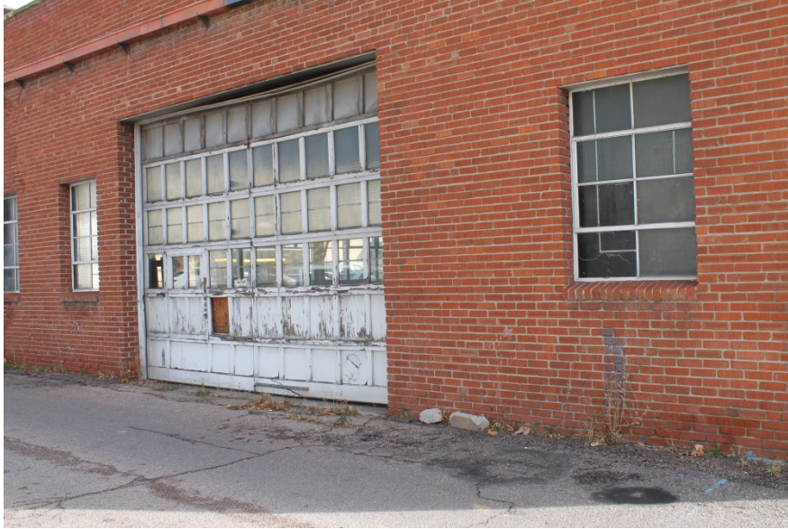
Figure 2-1 Deteriorated exterior walls and finishes; deteriorated windows and doors; deteriorated loading areas; presence of debris adjacent to structure; debris near high traffic areas; Inadequate site maintenance; non-conformance to development regulations; presence of debris next to structures (Photo 1)
