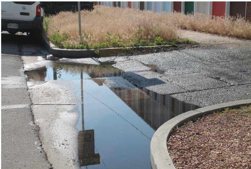
Figure 2-2 Cracked or uneven pedestrian surfaces; poor drainage; presence of trash and debris; potentially hazardous conditions; deteriorated drainage facilities; inadequate site maintenance; non-conformance to development regulations; debris near structures; fire hazards near structures; dead shrubs near high traffic areas; (Photo 2)
