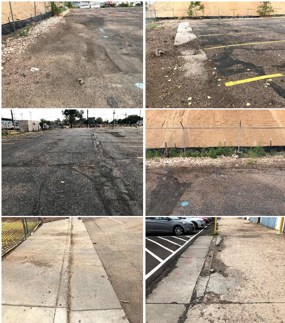
Figure 8. Deteriorated On-Site Parking Surfaces, Curb, & Sidewalks
