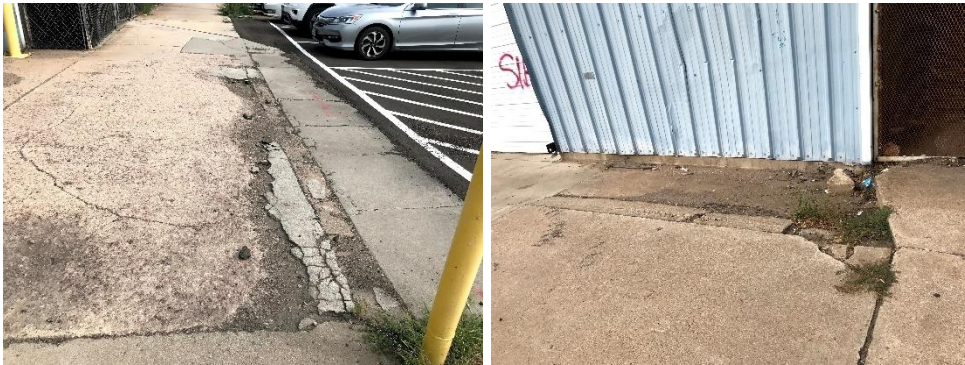
Figure 5. Cracked or Uneven Surfaces for Pedestrians
