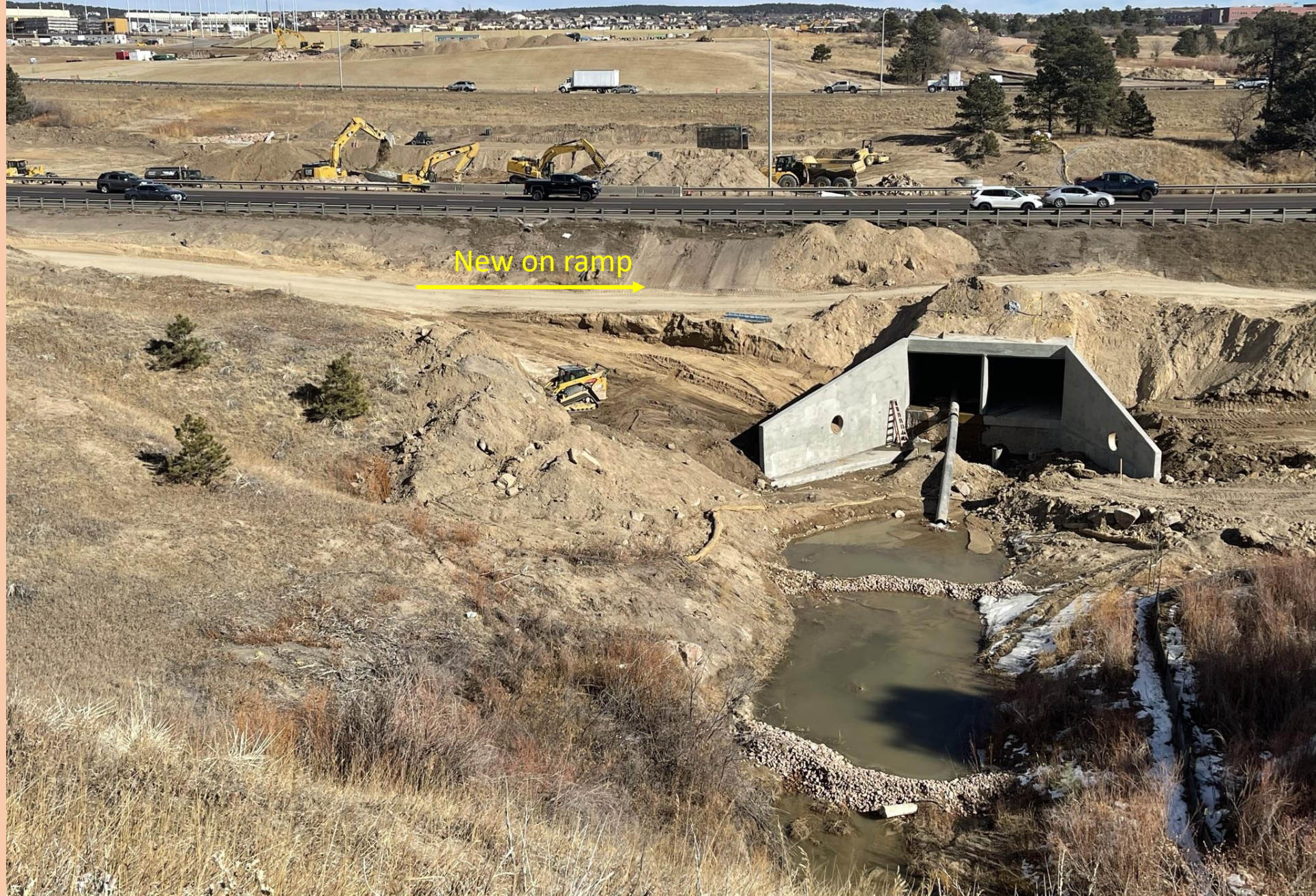
Looking east from Santa Fe Trail toward the box culvert extension, which will accommodate the southbound I-25 on ramp. Water Quality pond construction in the median
