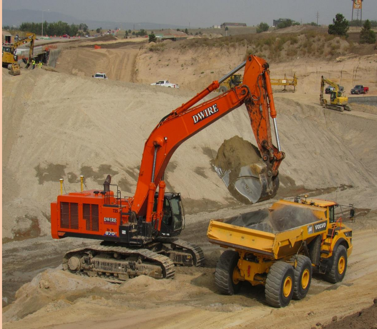
Over 1,500,000 CY of dirt has been moved by Dwire Earthmoving from Colorado Springs
