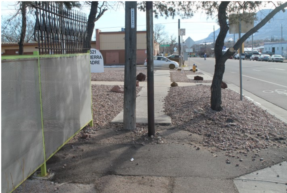
Figure 2-3 Substandard driveway/curb cuts, cracked or uneven pedestrian surfaces, unsafe level changes, deteriorated curb and gutter, inadequate and deteriorated sidewalk, non-conformance to development regulations (Photo A-9)
