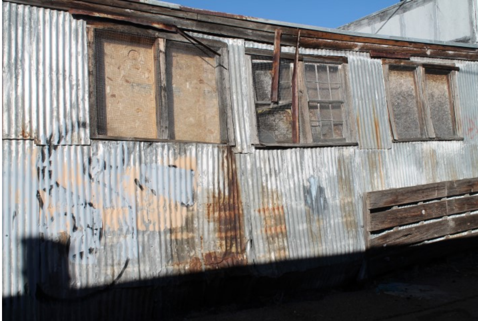
Figure 2-6 Multiple examples of deteriorated building exterior and structure, vagrants/vandalism/graffiti, building code violations (Photo B-16)
