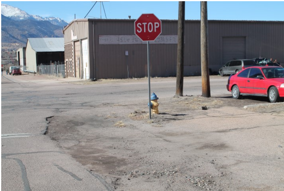
Figure 2-13 Poor vehicle access, lack of parking lot pavement, substandard driveway/curb cuts, cracked and uneven surfaces, unsafe level changes, deteriorated curb and gutter, inadequate and deteriorated sidewalk, non-conformance to development regulations (Photo E-4)
