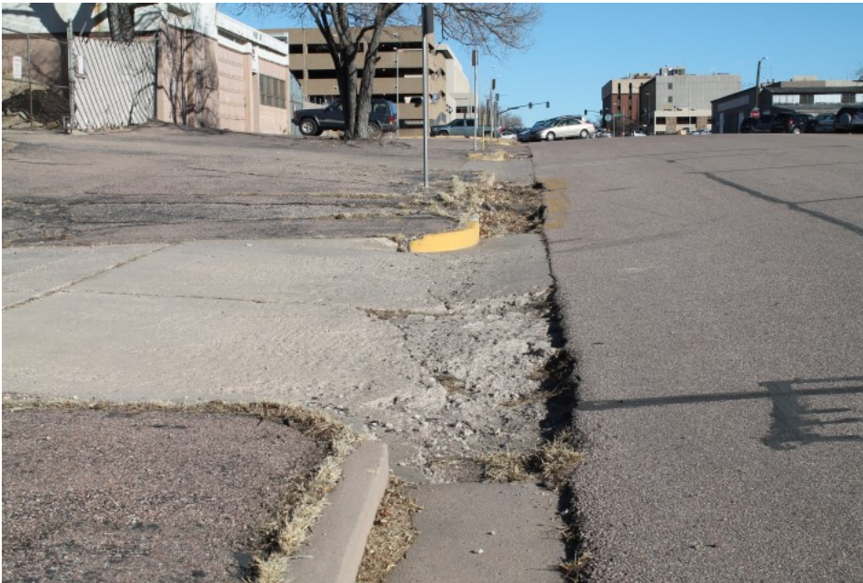
Figure 2-5 Presence of trash and debris, substandard driveway/curb cuts, cracked and uneven surfaces, unsafe level changes, deteriorated curb and gutter, inadequate and deteriorated sidewalk, inadequate site maintenance, non-conformance to development regulations (Photo B-11)
