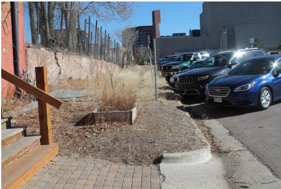
Figure 2-11 Poor vehicle access, substandard driveway/curb cuts, cracked or uneven pedestrian surfaces, unsafe level changes, inadequate and deteriorated sidewalk, presence of trash and debris, unsafe level changes, inadequate site maintenance, non-conformance to development regulations, deteriorated site walls (Photo D-10)
