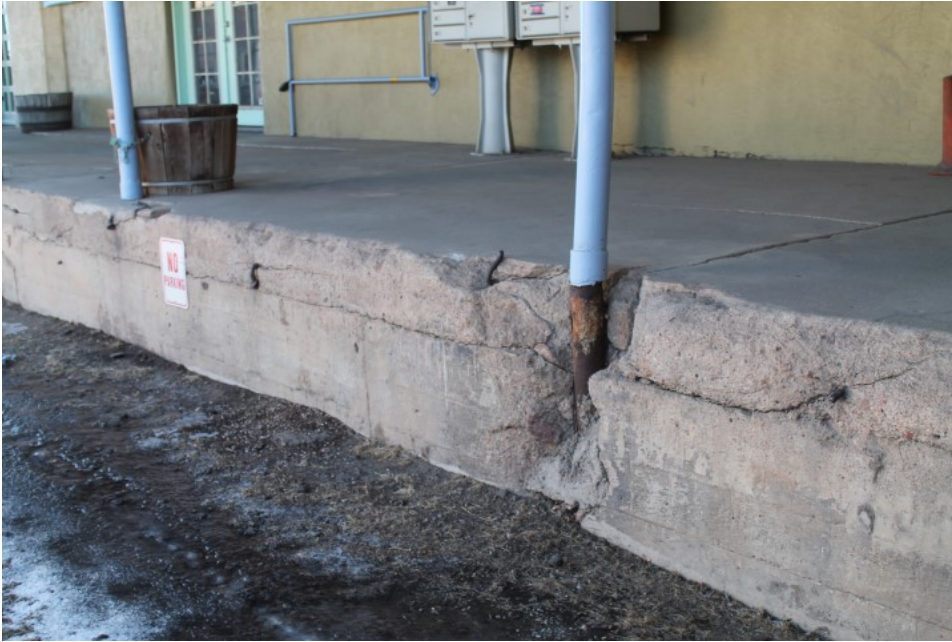
Figure 2-8 Deteriorated visible foundation, deteriorated gutter/downspouts, potentially hazardous conditions, unsafe level changes (Photo C-2)
