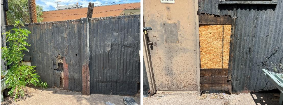
Figure 12. Deteriorated Fences and Walls
