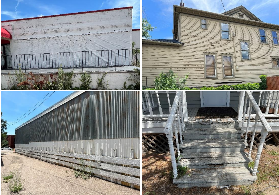
Figure 2. Deteriorated Exterior Finishes and Stairways
