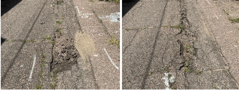
Figure 4. Poor Provision of Street Improvements for Vehicles
