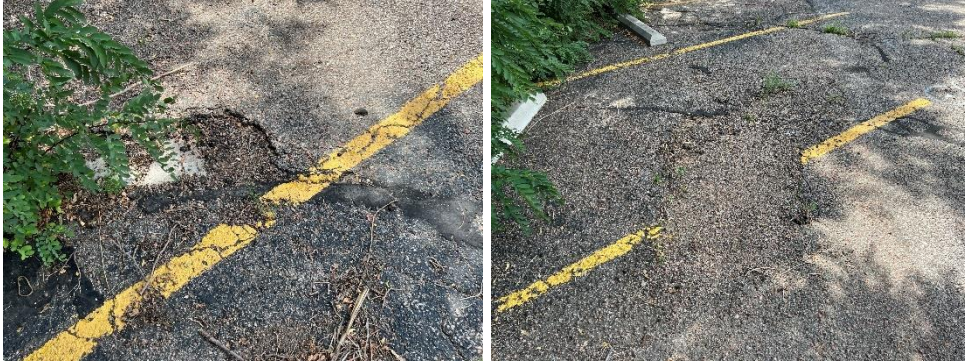
Figure 10. Deteriorated On-Site Parking Surfaces
