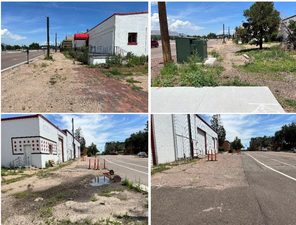
Figure 3. Poor Provision of Street Improvements for Pedestrians
