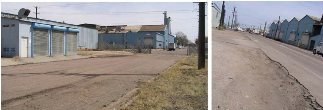
Exhibit 10: Condition F (Inadequate Public Improvements)
