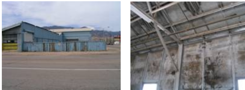
Exhibit 2: Examples of Condition A (Deteriorating Structures)
