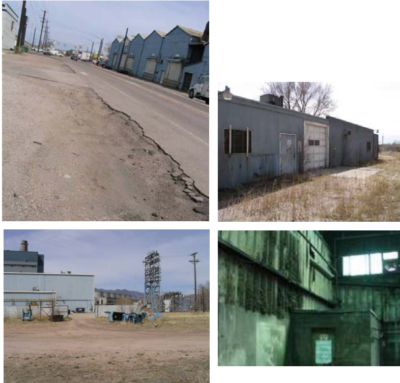
Exhibit 6: Examples of Condition D: Unsafe or Unsanitary Conditions
