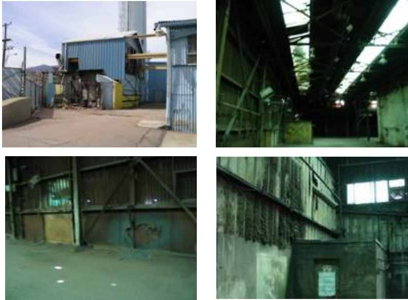
Exhibit 2 (cont.): Examples of Condition A (Deteriorating Structures)
